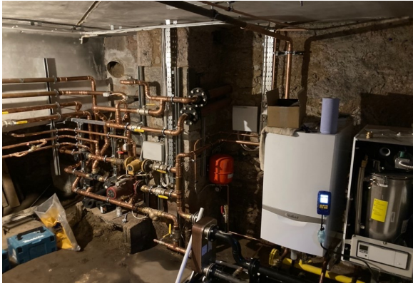
Boilers before insulation put on the pipes.
